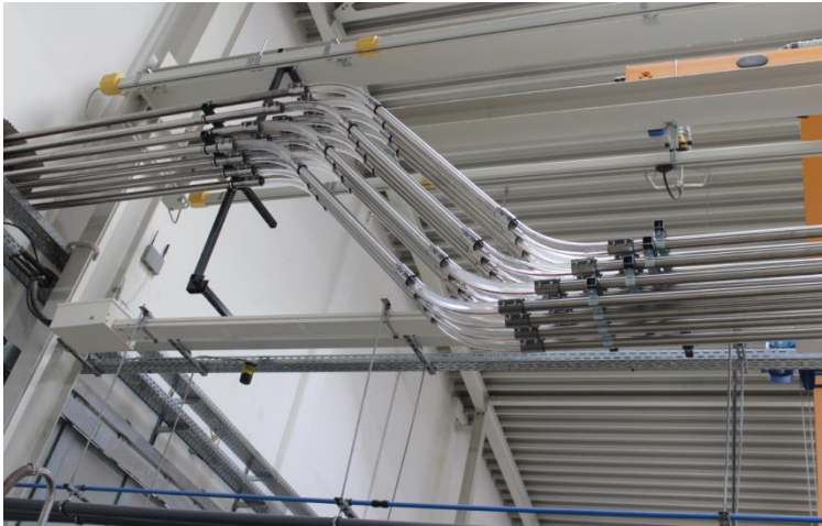
12 individual material lines from coupling station to 12 molding machines As well as the common material ring line for special material. Foto: Labotek
