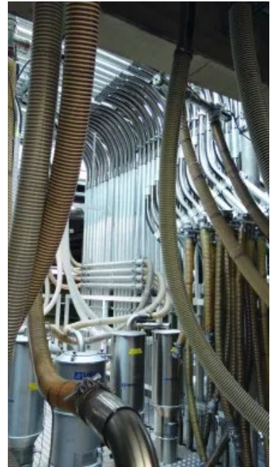
The granules reach the material stations via numerous pipelines. (Image: editorial team).
